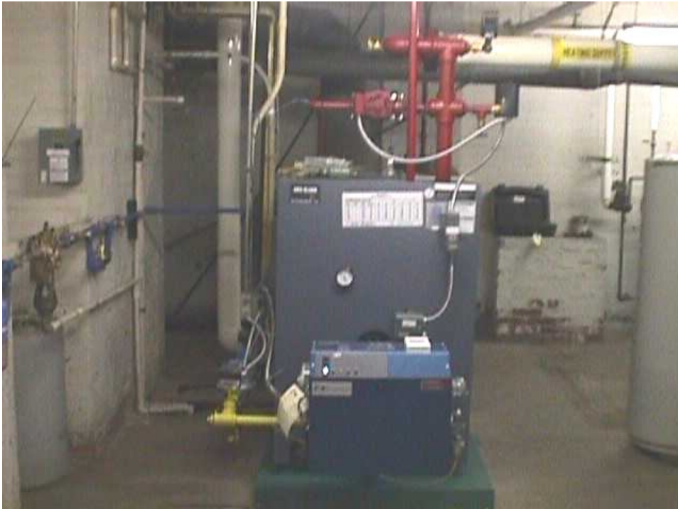
Photo of a newly installed boiler, Sept-2005. This is a 787,000 Btu input cast iron, Weil McLain boiler, equipped with a Power Flame burner.
